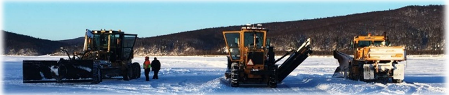
Aniak, Kalskag, and Napaimute Ice Road Crews Working Together for the Benefit of Everybody
